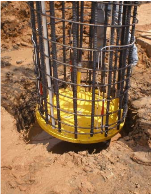
Grouting Cell at the base of the concrete reinforcement cage prior to installation deep into the ground.
